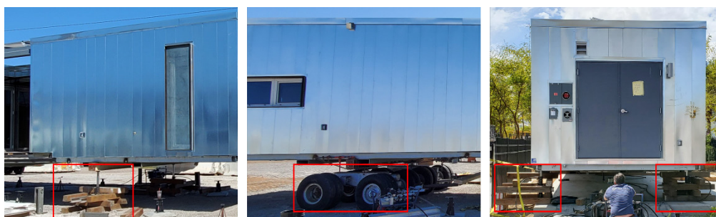
Figure 1. Lifting with hydraulic jacks (left), Transportation using tandem axle dollies (middle), Offloading with hydraulic jacks (right)
