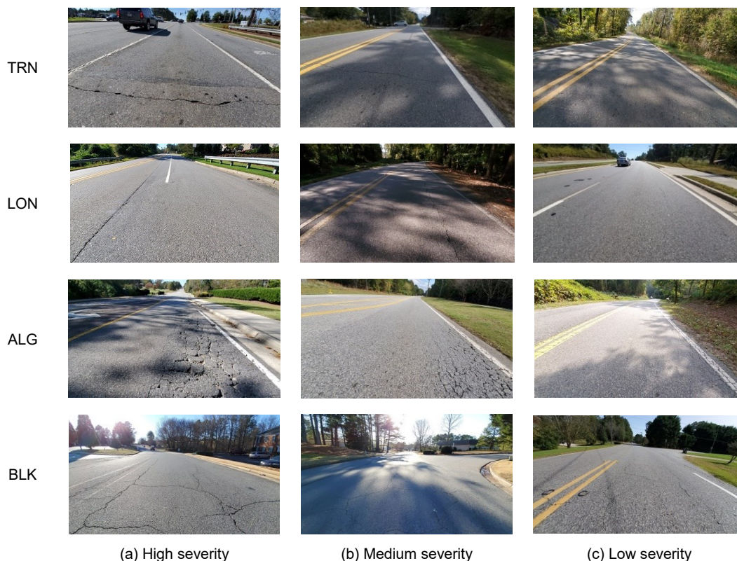
Fig. 2. Samples of some transverse, longitudinal, alligator and block cracks for three severities.
